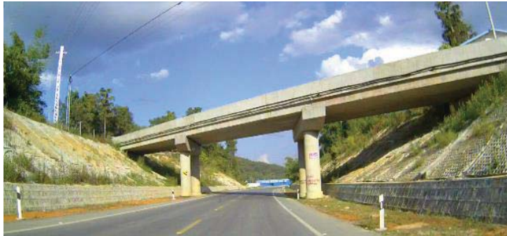
FIGURE 4.2.2.12 HIGHLY AGGRESSIVE UNGUARDED BRIDGE PIERS ( driving is on the right side of the road )
