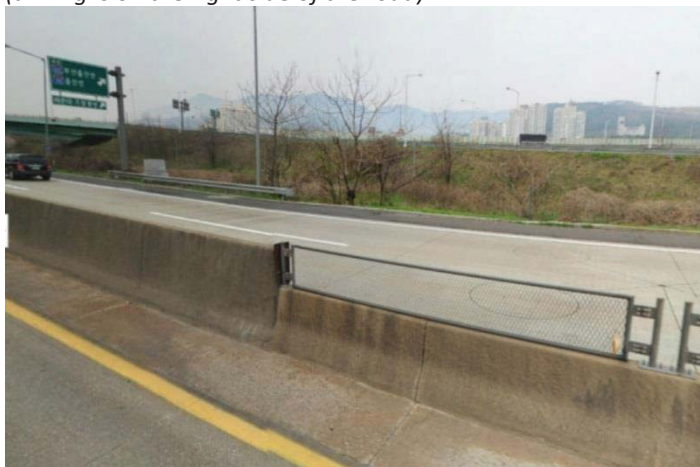
FIGURE 6.2.3.5 1270MM HIGH CONCRETE SAFETY BARRIER AS ANTI-GLARE SYSTEM (driving is on the right side of the road)
