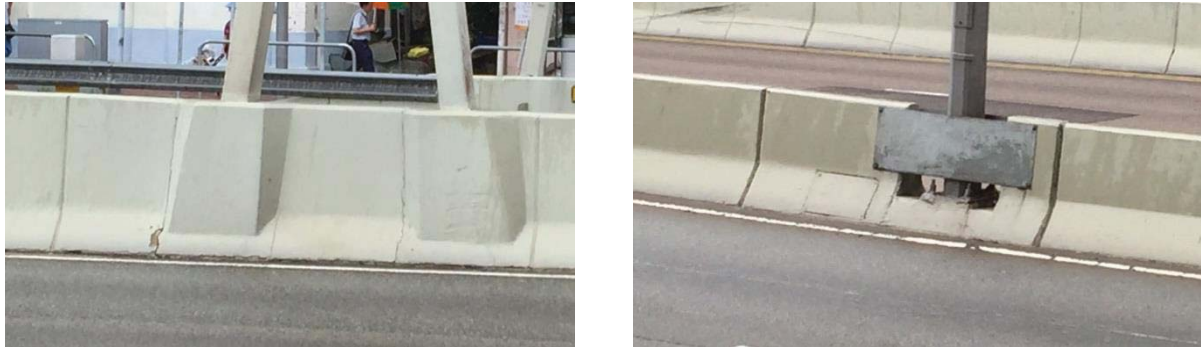
FIGURE 4.3.2.5 TYPICAL DEFICIENCIES OF SAFETY BARRIERS
