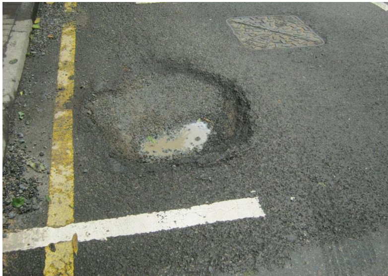
FIGURE 2.5.3.1 A POTHOLE ON THE CARRIAGEWAY
