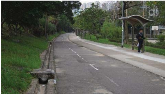
FIGURE 5.3.1.3 ROADSIDE HAZARDS ALONG A BICYCLE TRACK ( cycling is on the left side of the road )
